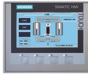
Touch Screen PLC (pic.2)
